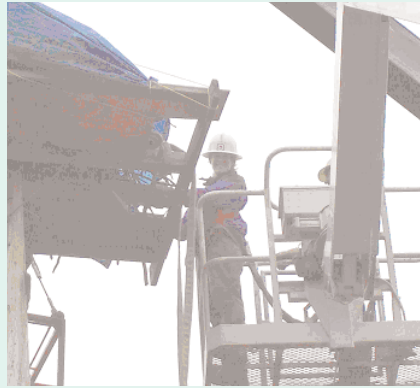
Husky's Carol Engstrom putting a tarp over the nest prior to moving the pole
